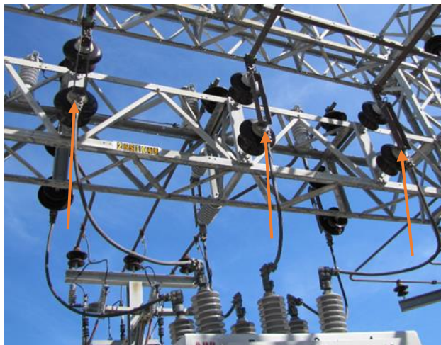
Figure 5: Example of disconnect switches to be replaced
