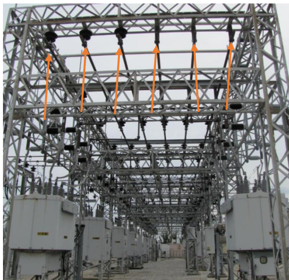
Figure 4: View from North side of structure, example of bus insulators to be replaced
